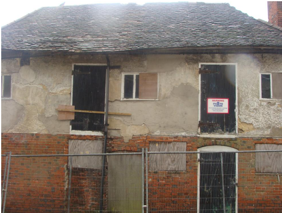
Picture 738. Outbuildings rear of no.12 North Street- a building identified as being 'At Risk' but one where works had commenced in 2013.
