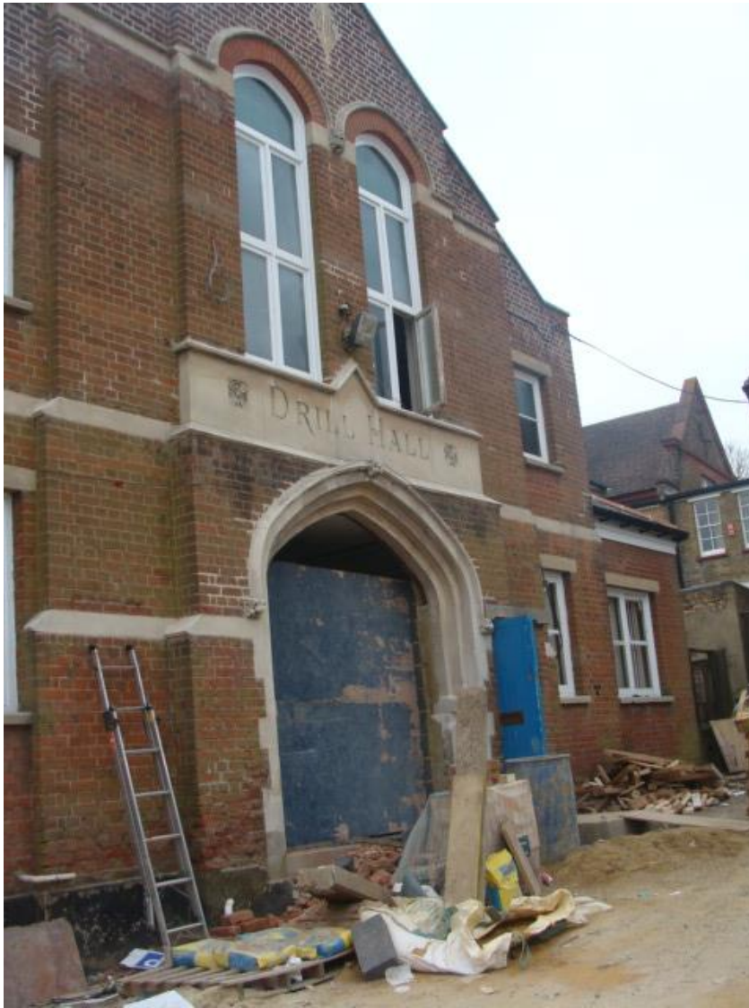
Picture 89. The former Drill Hall, now being converted to a restaurant. It is important that stone detailing is retained.
