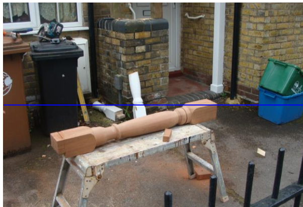
Pictures 69 and 70 Kings Cottages, the Conservation Area is proposed to be extended to include these two groups of early 20 th century cottages of quality and historic interest. Lower picture shows properly turned wooden replacement support being fitted, being an exact copy of the original.
