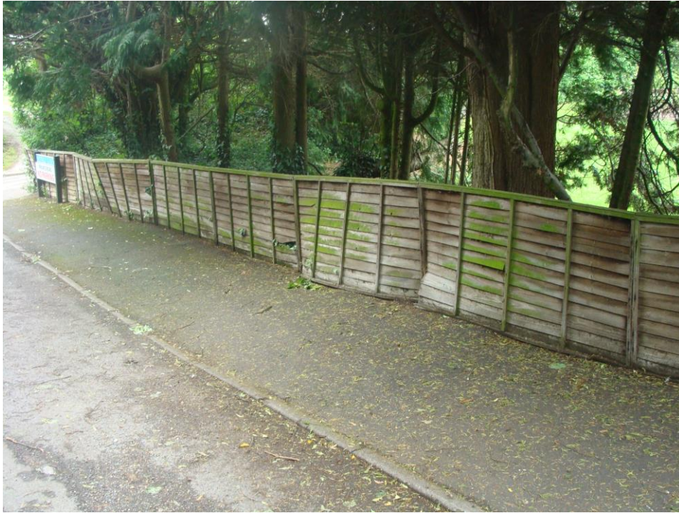
Picture 175. Deteriorating fence to front of Snowlands. This may need replacing in the future; an ideal solution would be with railings or hedge.
