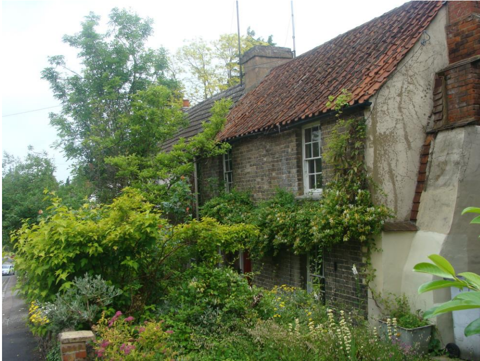
Picture 8377 . Nos. 10-12 Bell's Hill. Pair of non listed cottages worthy of retention. Some repair works to roof have been carried out.
