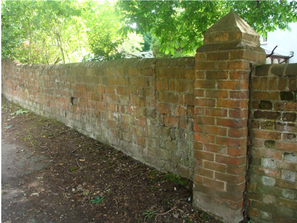
Picture 143. Boundary wall, east of no. 86 Hadham Road. Walls are a feature of the town in this area and need to be retained. Note unusually large brick sizes of this example.
