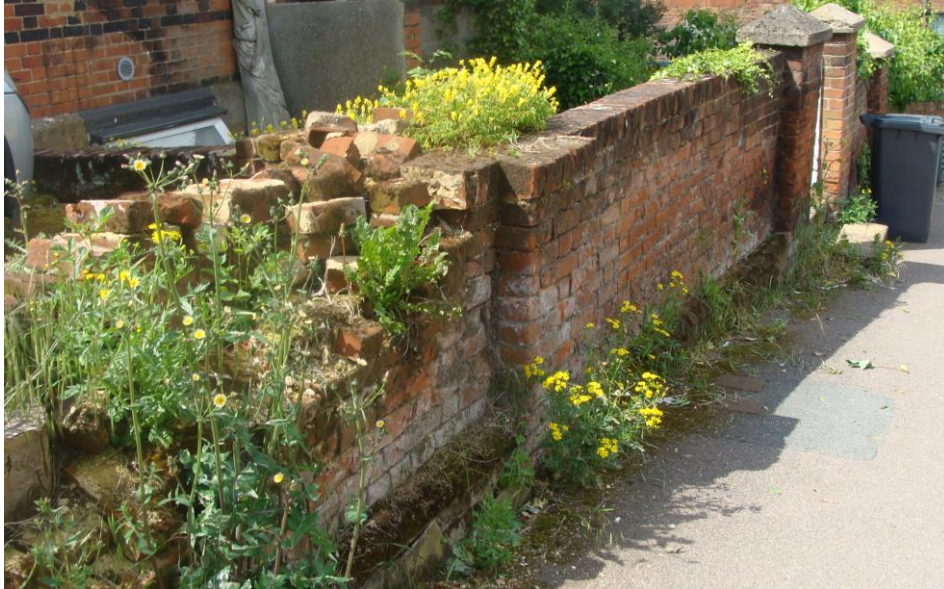
Picture 4237. Wall at Grange Road in urgent need of repair.
